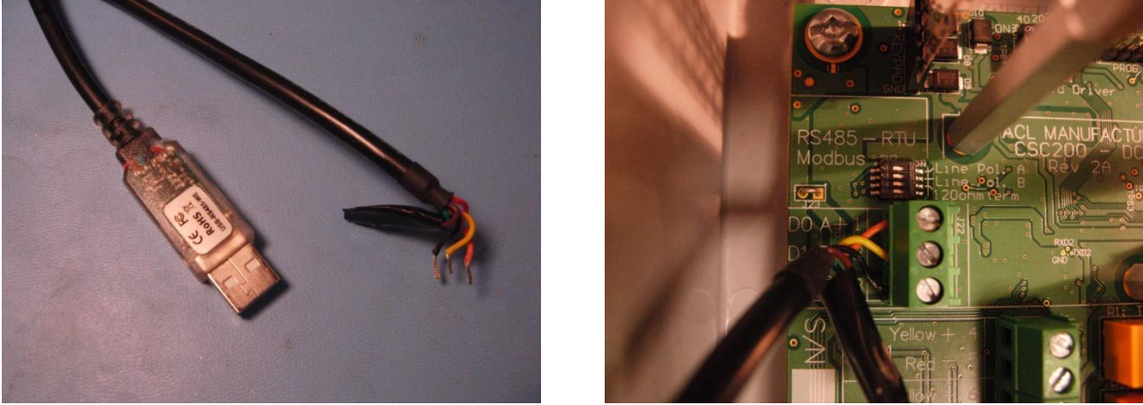
Figure 5 - FTDI Chip USB-RS485-WE-5000-BT USB to RS485 Cable, Installed with CSC400 Controller
